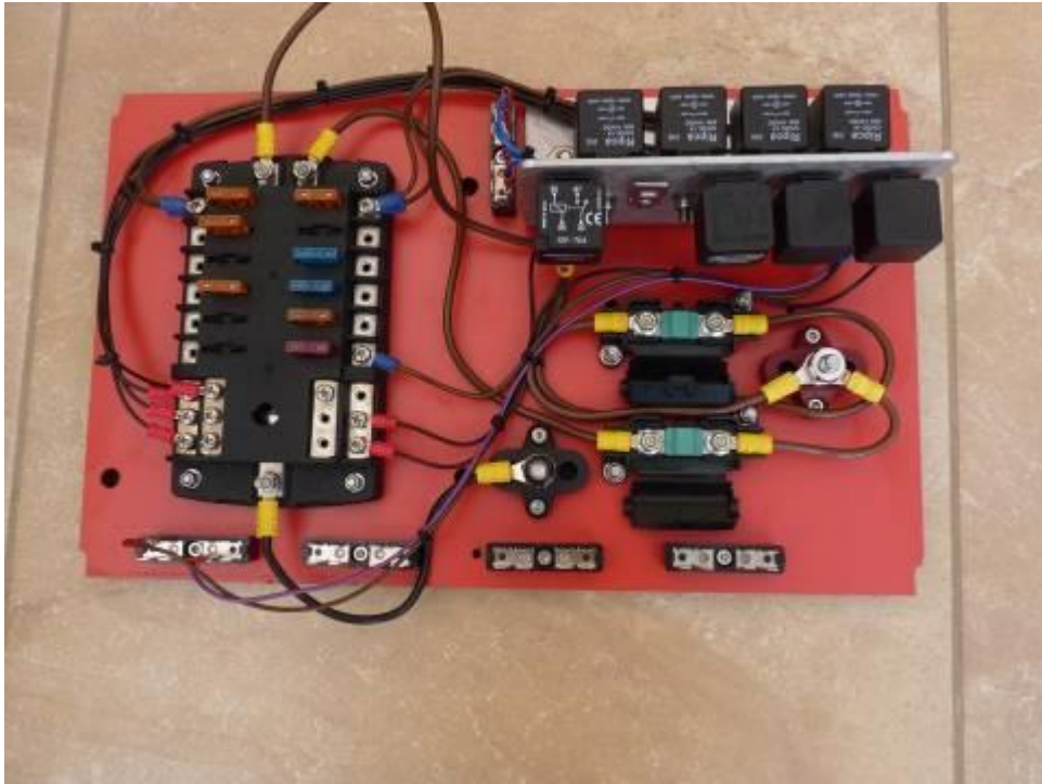
Kermit's electric panel.
